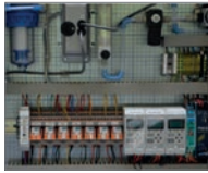
Equipment for inertization of the testing area
