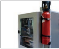
CO 2 fire suppression equipment
